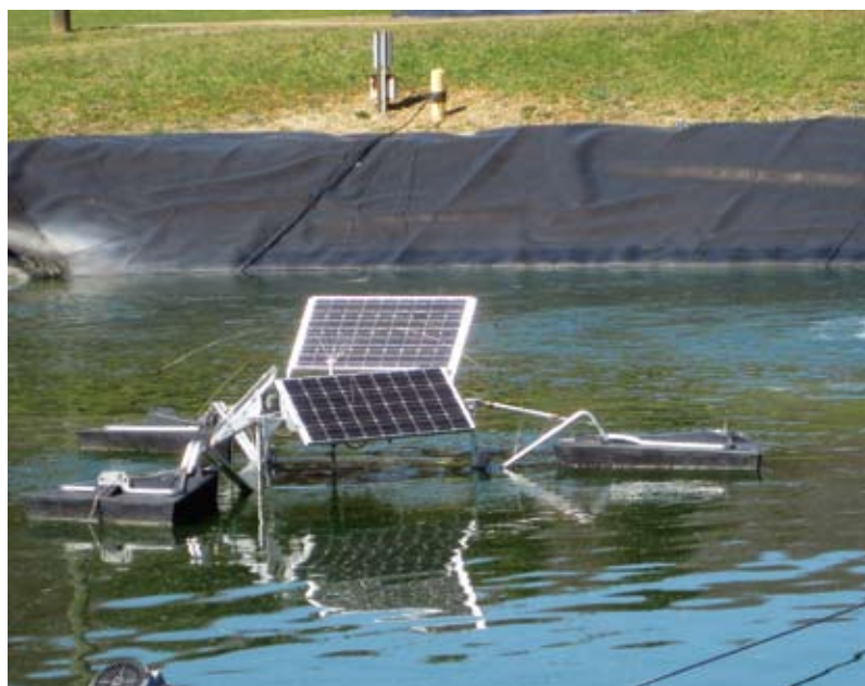
The township installed three solar-powered units in 2009, reducing electricity consumption.
