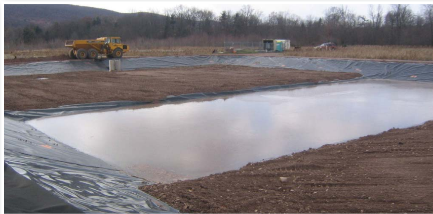
Free water wetlands beds with deeper re-aeration zone.
